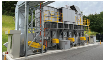
Introduction of energy-saving equipment (thermal storage deodorizers): Nissha Industries, Inc. (Japan)
