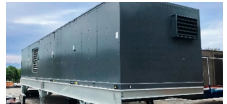
Energy-saving equipment (HVAC) to be installed: Nissha Medical Technologies (USA)
